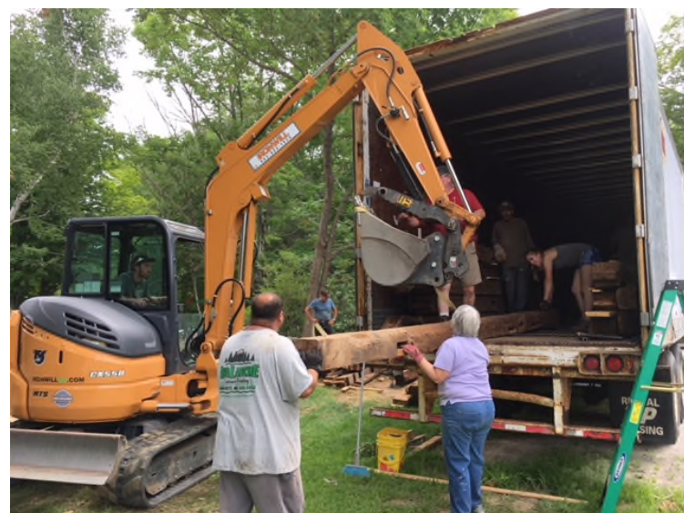
Volunteers loading timbers into trailer. Ironwill Contractors donated use of their equipment and operator. Burley Chamberlin, operator.
